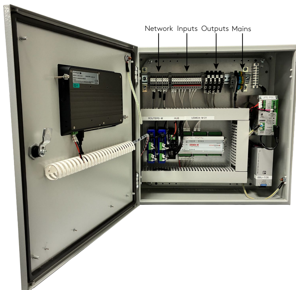
Figure 4. Wiring Inside the Control Panel
